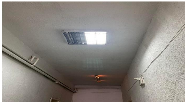
Figure 8 The lights and their damage are not the same.
