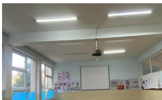
Figure 4. The lighting is damaged
